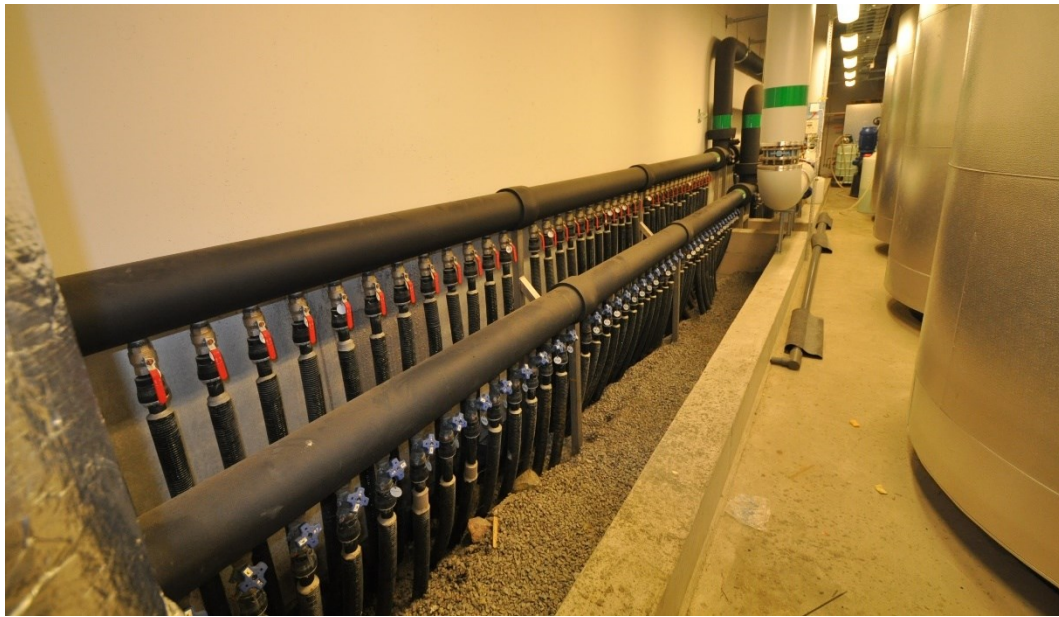
Figure 7-8: Piping to Boreholes in the Energy Central
