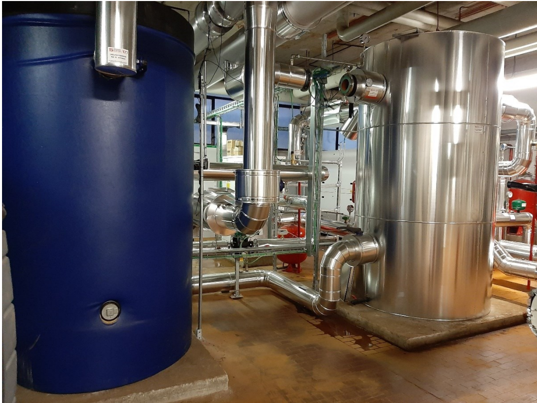
Figure 6-13: View of the Municipal building substation
