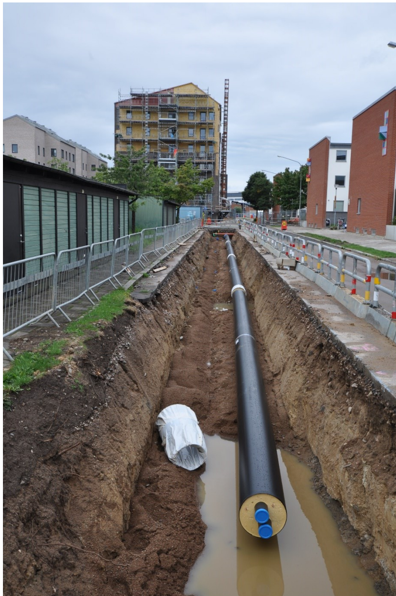
Figure 4-6: District Heating Piping
