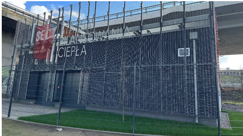
Figure 8-6: Heat Balancing Station
