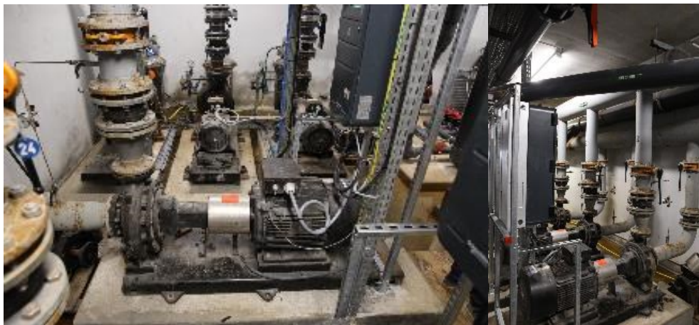
Figure 5-7: Variable speed pumps in the pumping station. Source: EDF.
