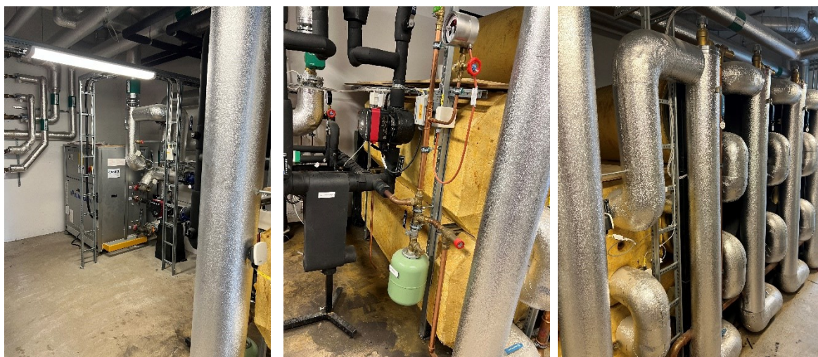
Figure 7-11: Booster Heat Pump installed at the Hotel (left); Heat Exchanger to the Local DH Network at the Hotel (centre); Piping to 10 TES in Series (right)
