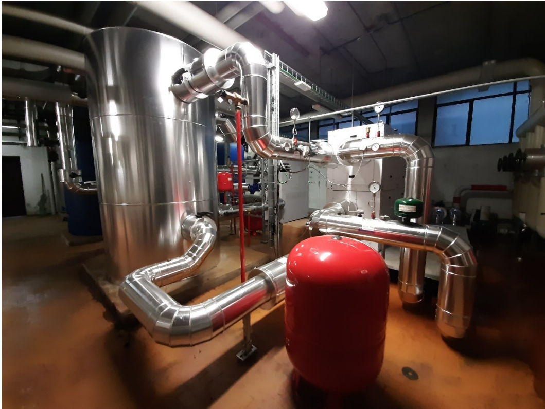
Figure 6-11: View of the central distribution substation
