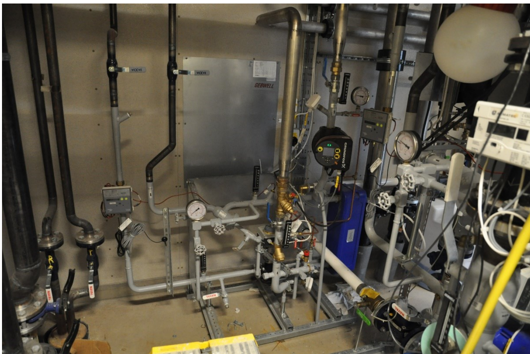
Figure 4-10: Heat Exchanger for Boreholes
