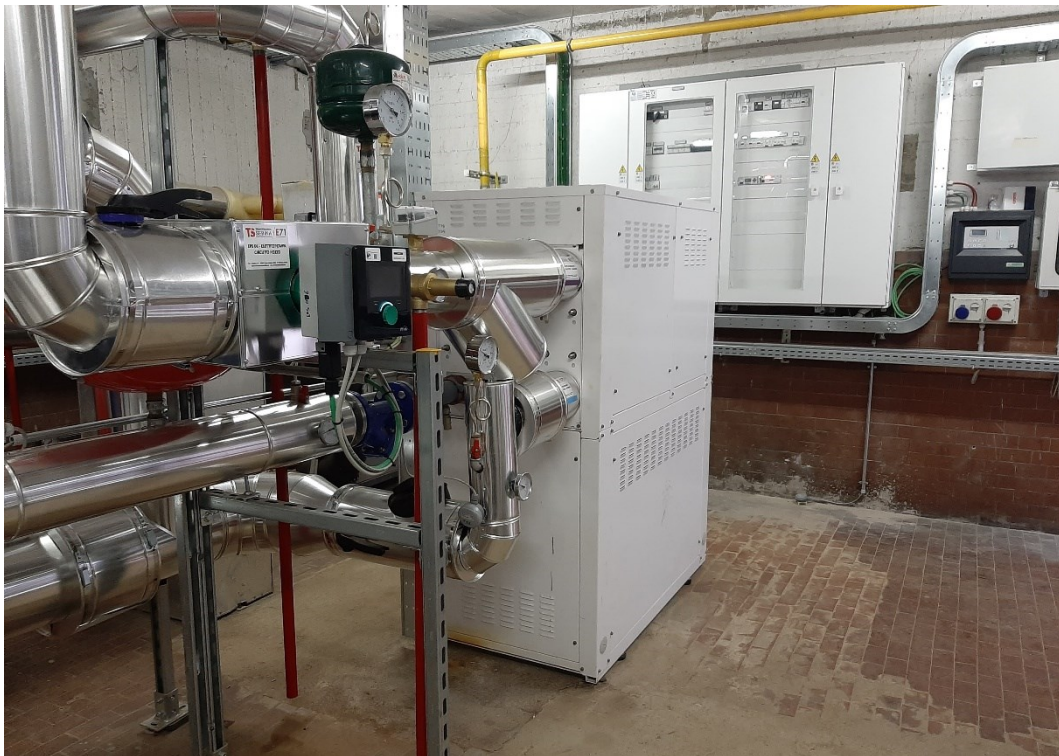
Figure 6-12: View of the Municipal building substation
