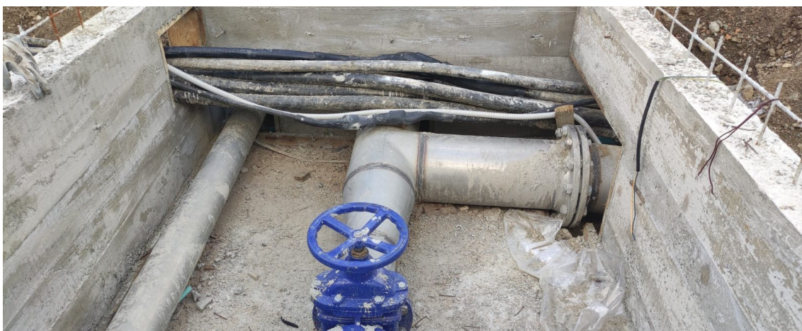
Figure 9-11: The main inlet of geothermal water in CTS from source TEB-4
