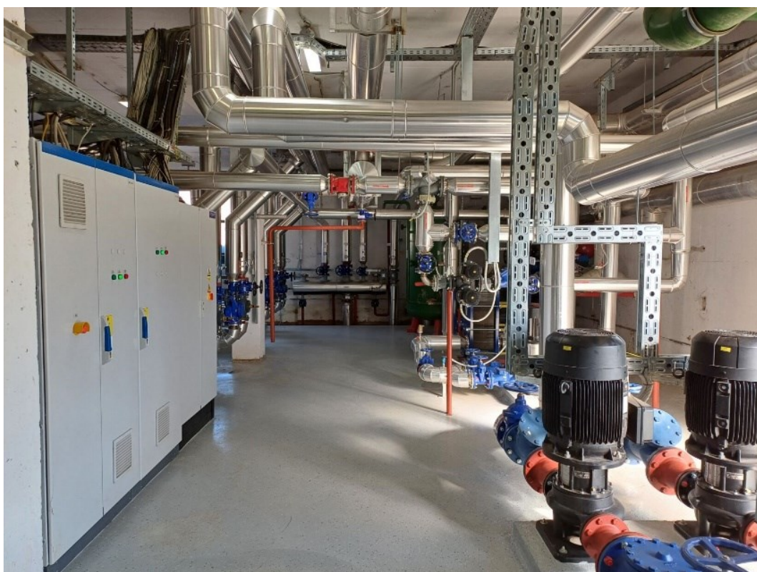
Figure 9-16: CTS new floor, electrical cabinets and equipment
