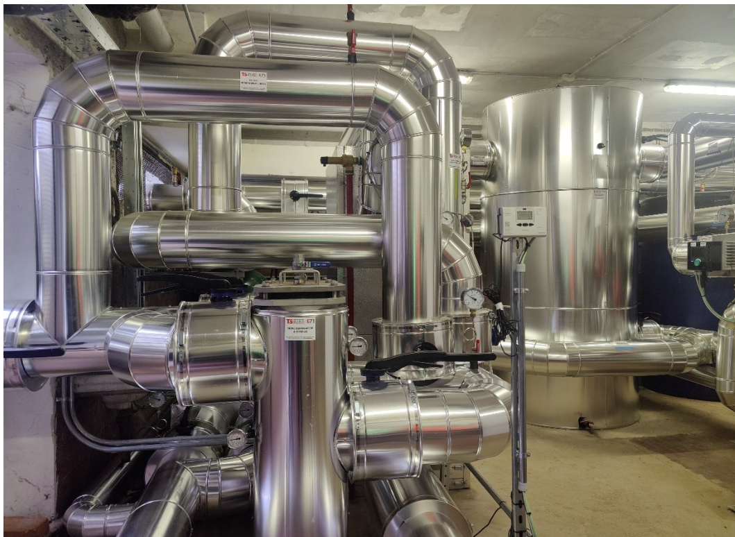
Figure 6-10: View of the central distribution substation
